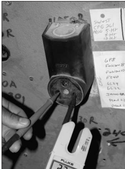
Checking the voltage of a wall outlet.
