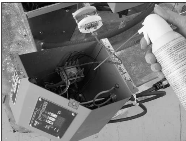
Whenever you open the switch box, blow out the dust with canned air.
