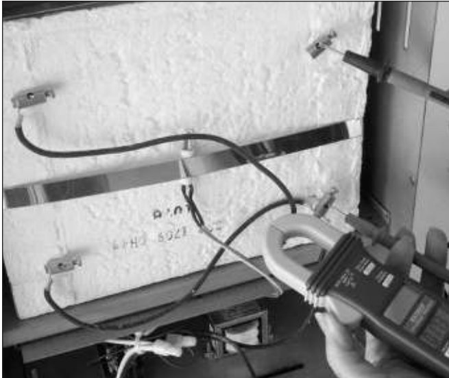
Shown here is a 120 volt SC-2 kiln that has two elements wired in parallel. Note that the two wires have been disconnected from the upper right element connector before testing with an ohmmeter.
